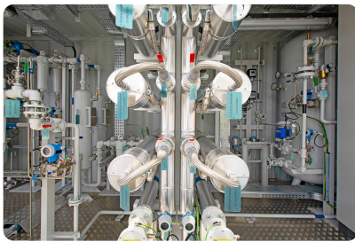
NITROGEN GENERATION - MEMBRANE TECHNOLOGY - Sinergia.
